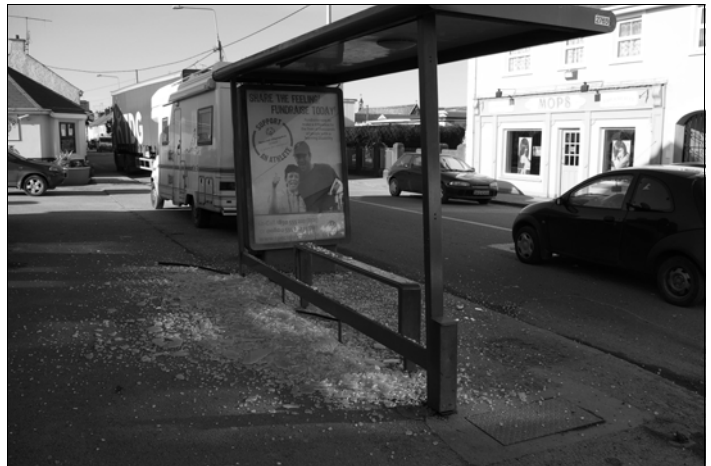
The bus shelter outside the Community Centre was hit by a vehicle on January 25th. The vehicle did not stop.
